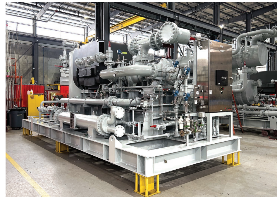
Refrigeration Package - Mayekawa USA 3225SSC / 1000HP
