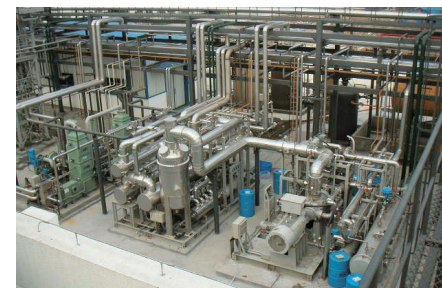
NH 3 Recovery / Purification Plant - China 2520SSC / 280kW
