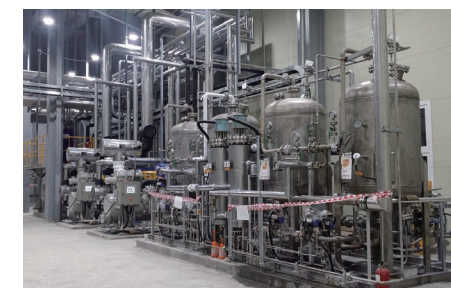
CO 2 Liquefaction Plant - Korea 200S / 230kW
